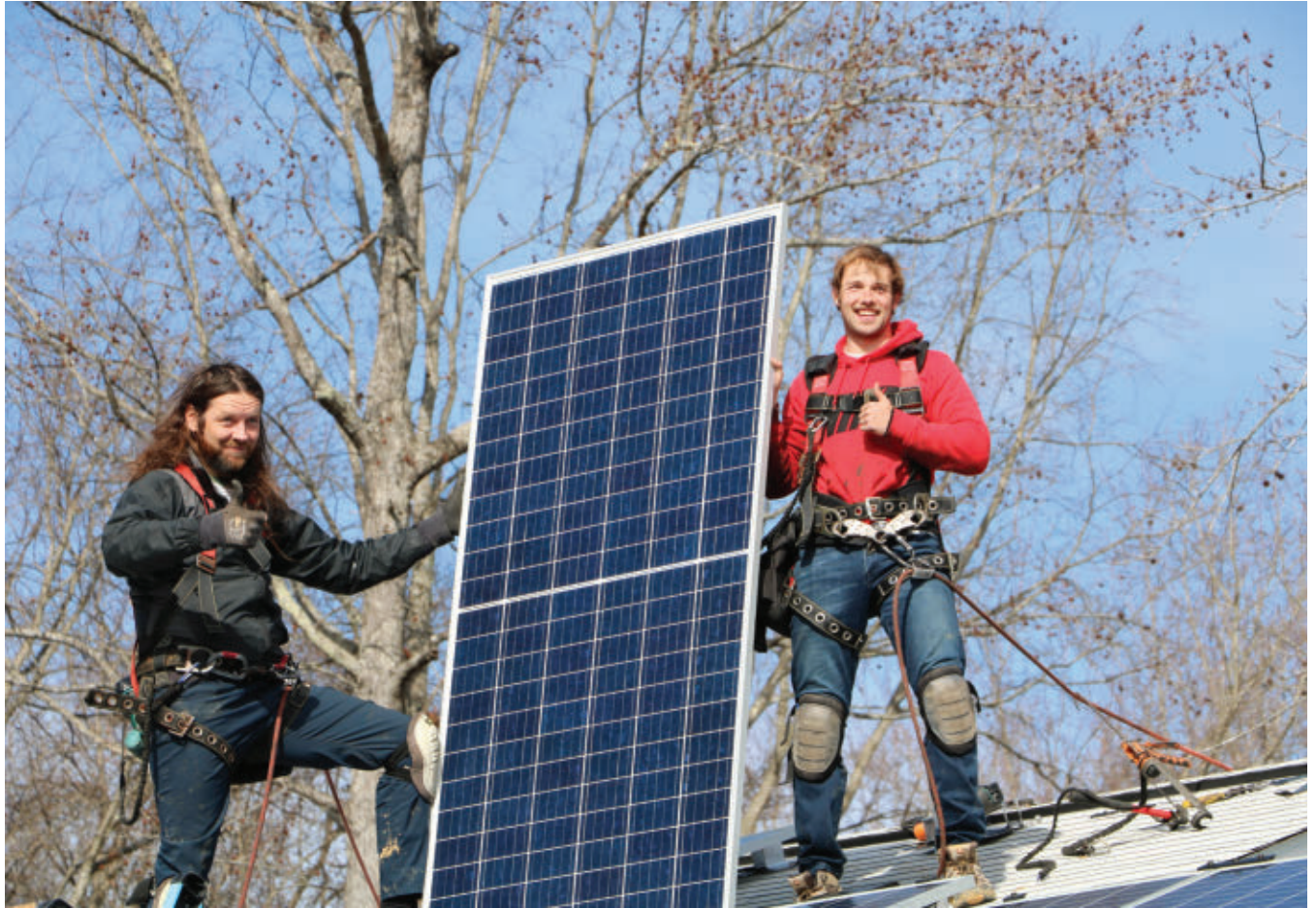
Workers install solar panels on the roof of a Habitat for Humanity home in Hillsborough, North Carolina.
