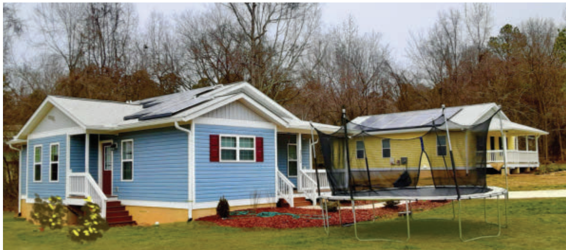
Left: Homes built by Habitat for Humanity with rooftop solar panels in Orange County, North Carolina. Bottom: Volunteers lift a solar panel during installation at a Habitat home in Harrisonburg, Virginia.
